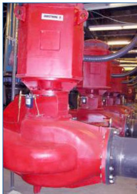
Enwave District Cooling Facility, Toronto, Canada.
