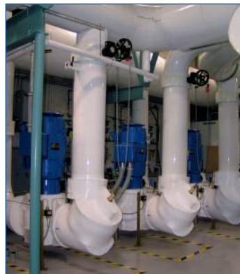
District Cooling Project, Phoenix, U.S.A.
